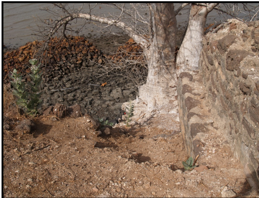
Figure 12. North wall of southeast bastion showing significant collapse and baobab tree growing at the base (photograph by author).
