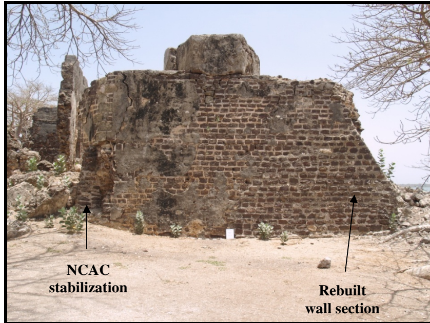
Figure 11. East wall of southeast bastion showing NCAC rehabilitation efforts (photograph by author).
