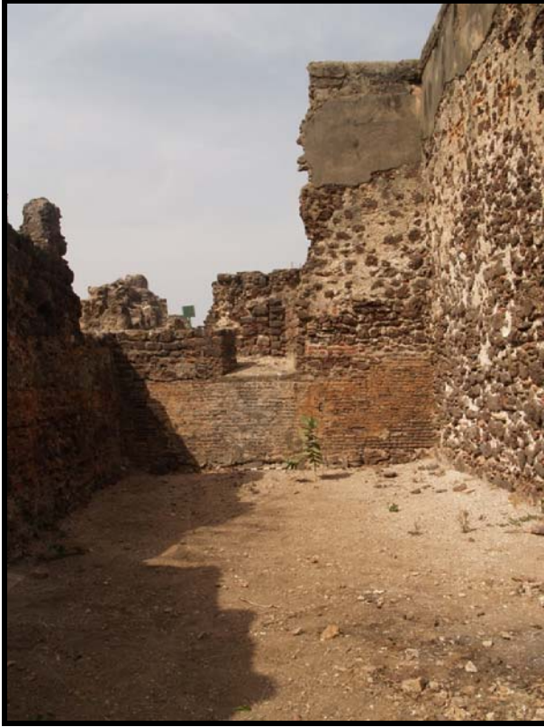
Figure 7. Lower level western apartments showing the absence of internal wall taken from the south (photograph by author).
